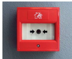
Fire alarm call point
