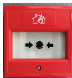
Fire alarm call point
