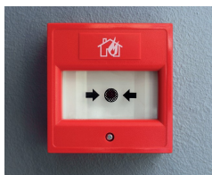
Fire alarm call point
