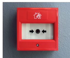
Fire alarm call point
