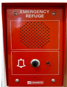
Commend refuge communications intercom
