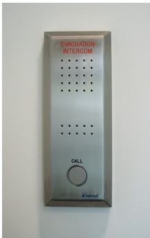
Windcrest refuge and lift communications intercom
