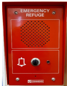
Commend refuge communications intercom
