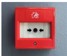
Fire alarm call point
