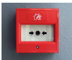
Fire alarm call point
