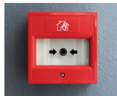
Fire alarm call point
