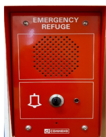
Commend refuge communications intercom
