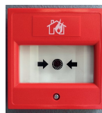
Fire alarm call point
