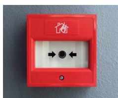
Fire alarm call point
