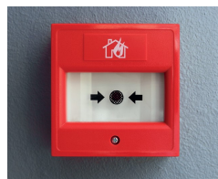
Fire alarm call point
