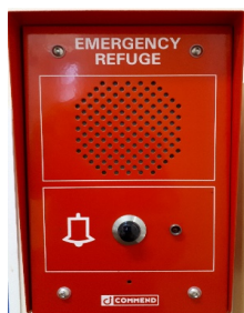
Commend refuge communications intercom
