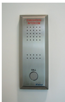
Windcrest refuge and lift communications intercom
