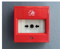
Fire alarm call point
