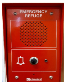
Commend refuge communications intercom
